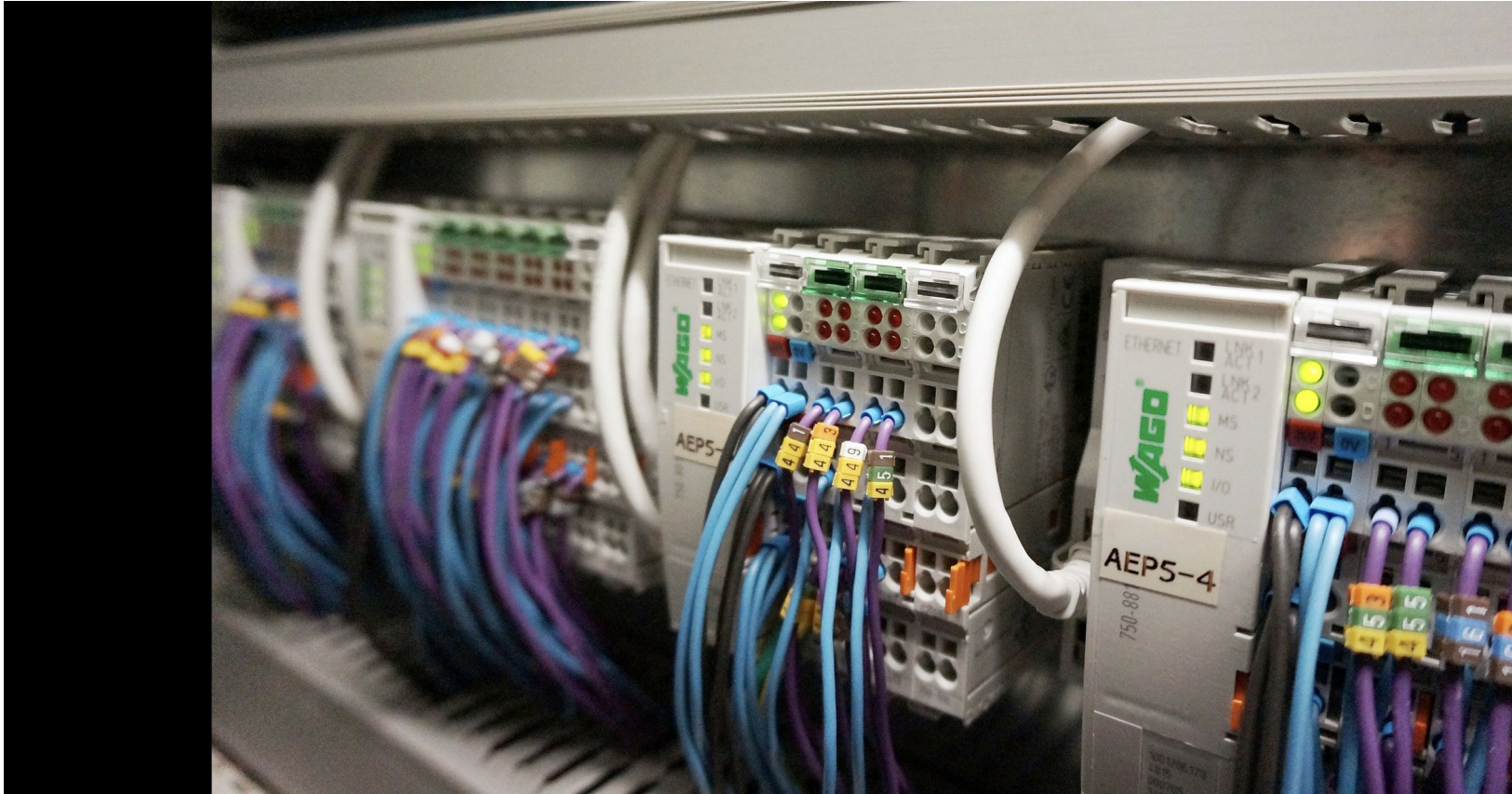
PLCs for a monitoring system in the pharmaceutical industry
